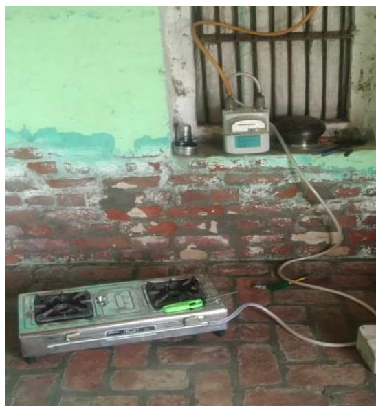
Fig. 3. Installed Biogas flowmeter at village dholu plant
